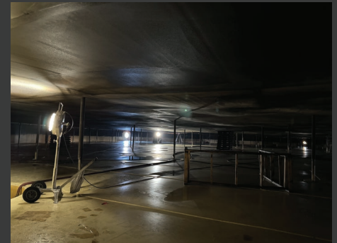
Clean for Inspection
